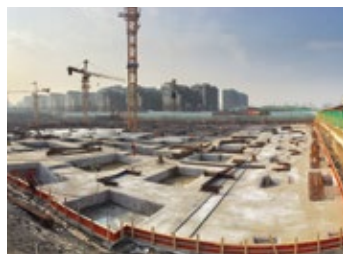
Broke ground for the Nanjing International Water Hub on the Sino-Singapore Nanjing Eco Hi-tech Island in March. Construction is progressing well, with completion targeted for 2018
